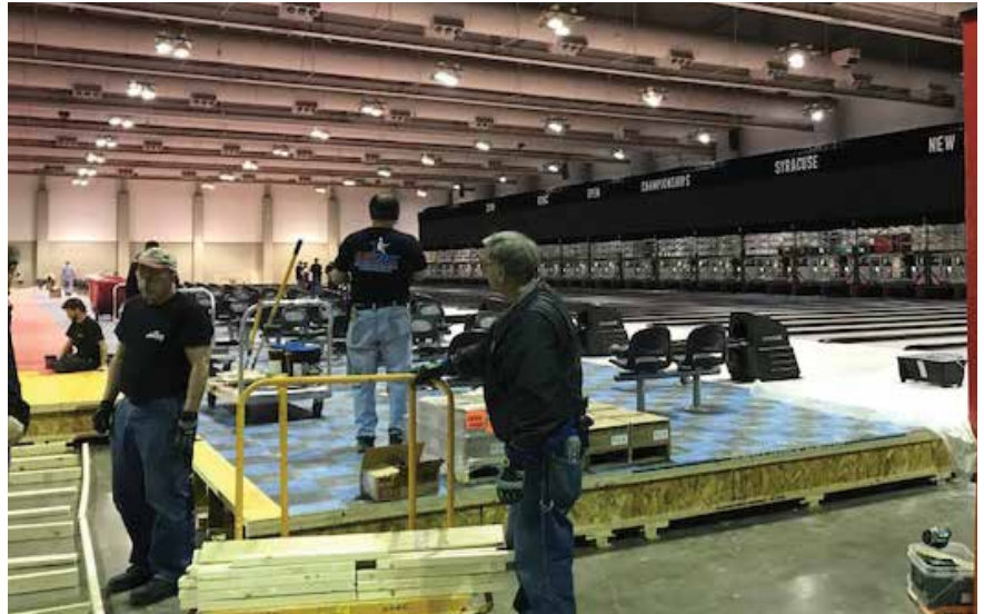
Workers build 48 bowling lanes, thereby converting the Convention Center at Oncenter into a state-of-the-art championship bowling venue.
