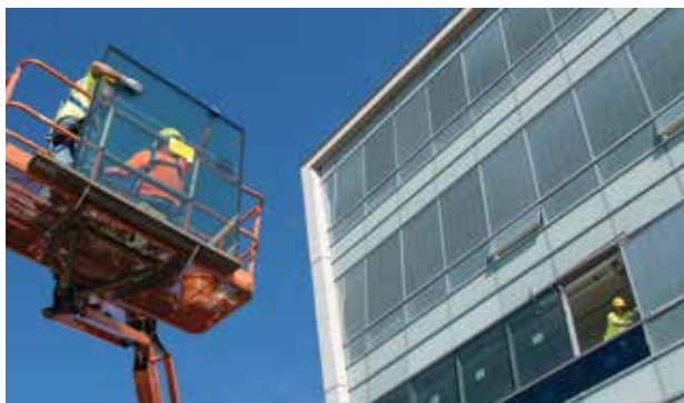
Electrochromic windows are installed at the SyracuseCoE to study the quality of daylight and how it impacts office workers.
